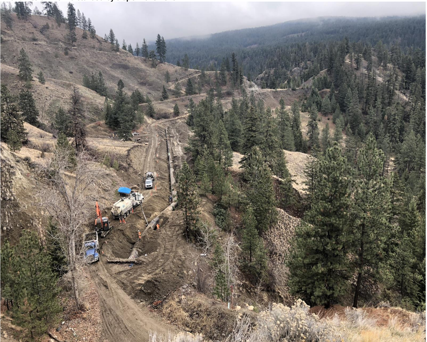
Transmission Main disturbed by slope movement.
