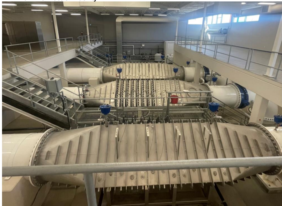
BMID UV Disinfection Facility
