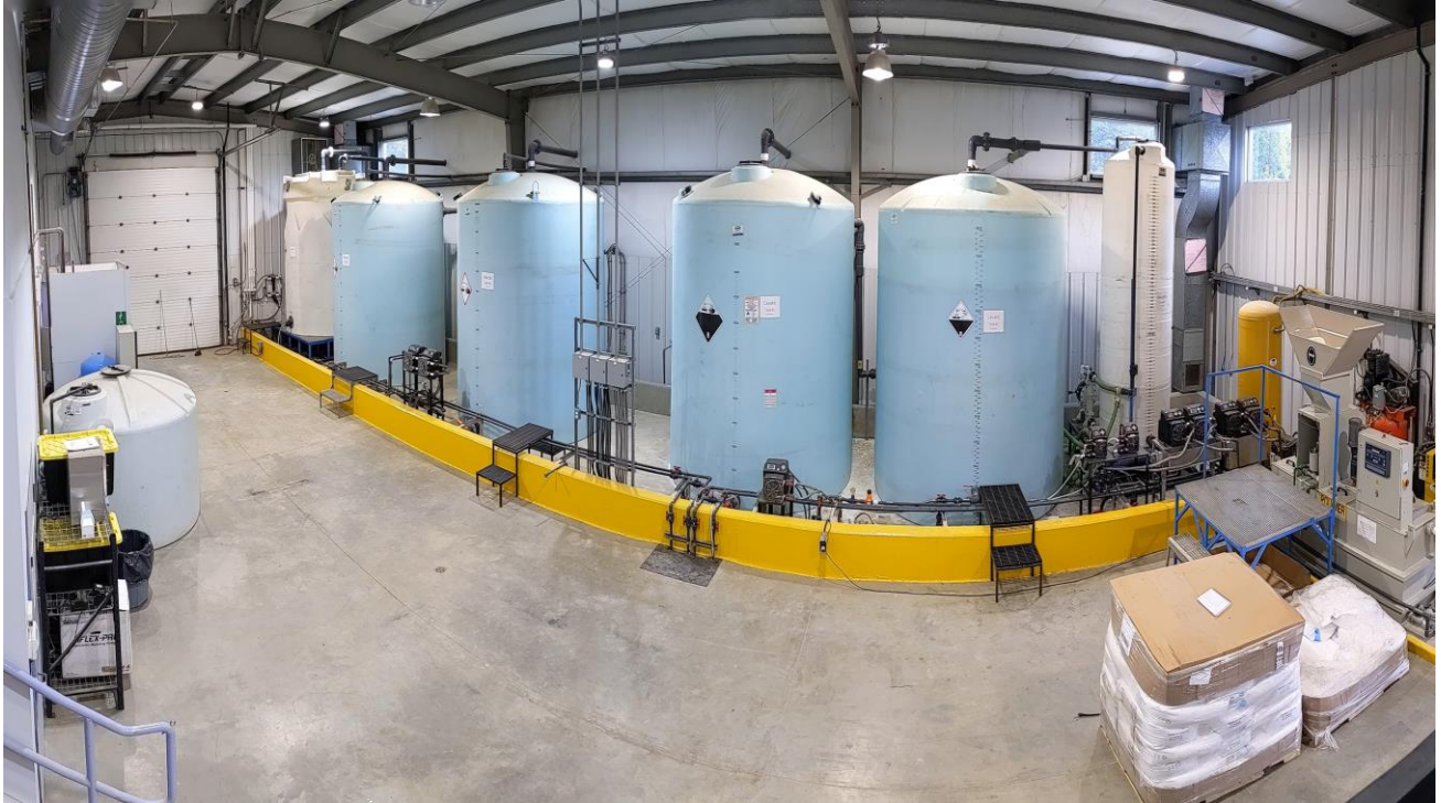
Chemical tanks at the Water Treatment Plant Operations building
